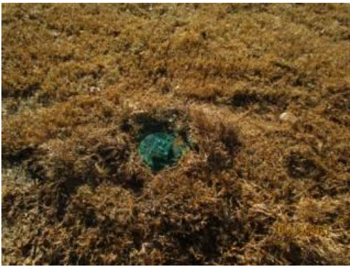
Photo X-55 The cleanout is located in the front yard.
