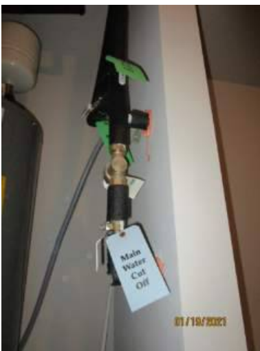
Photo X-53 The main water shut off is located in the garage
